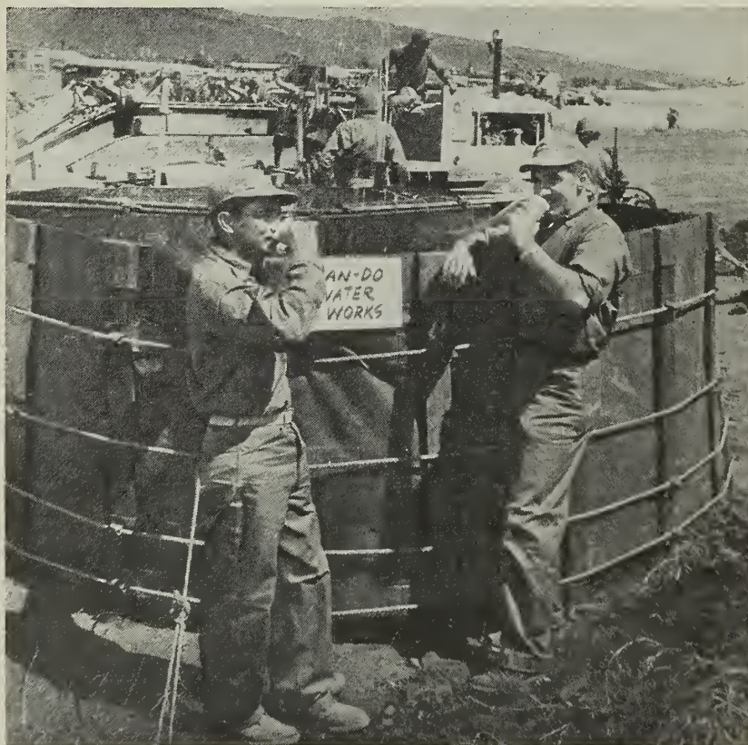
THIRST QUENCHERS —Setting up an advanced base can include problems such as building water-purifying systems like these Reservists have made.
